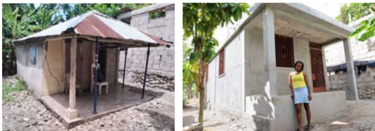
Before (left) and after (right) Build Change technical and financial support for repair and retrofit of Naomie Gobert's home
