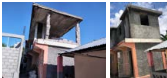
Before (left) and after (right) Build Change technical and financial support for repair and retrofit of Aurore Medard's home
